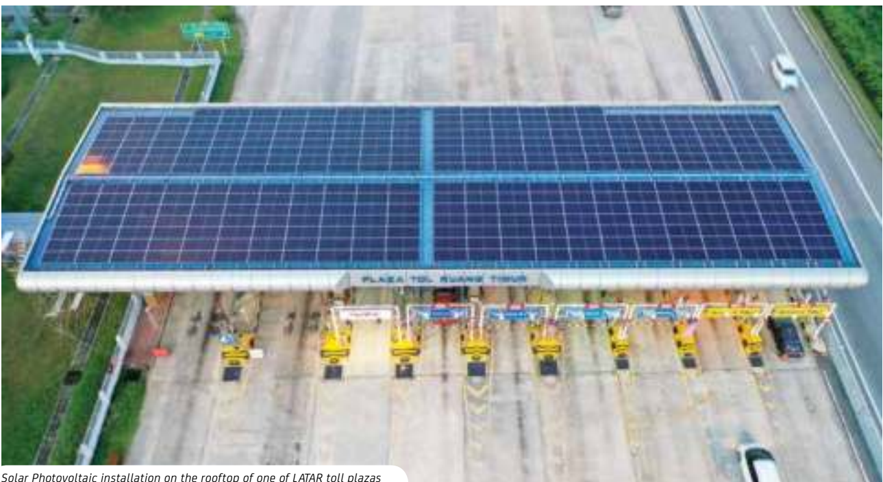
Solar Photovoltaic installation on the rooftop of one of LATAR toll plazas
